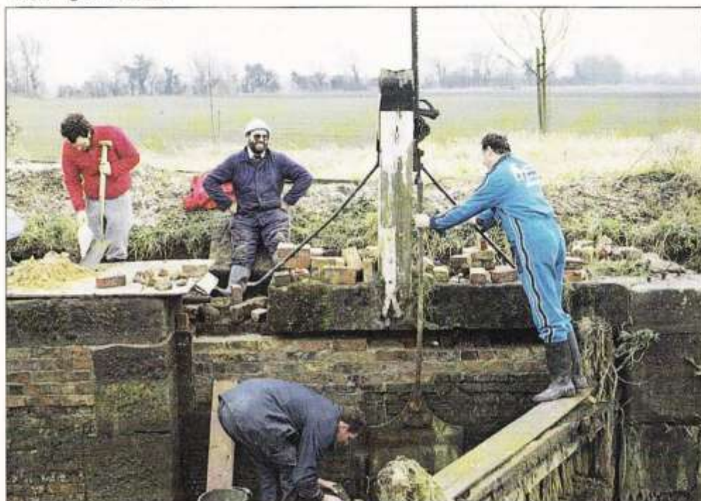
Below – Volunteers carry out repairs to the upper gate recess at Top Lock on the Pocklington Canal.
