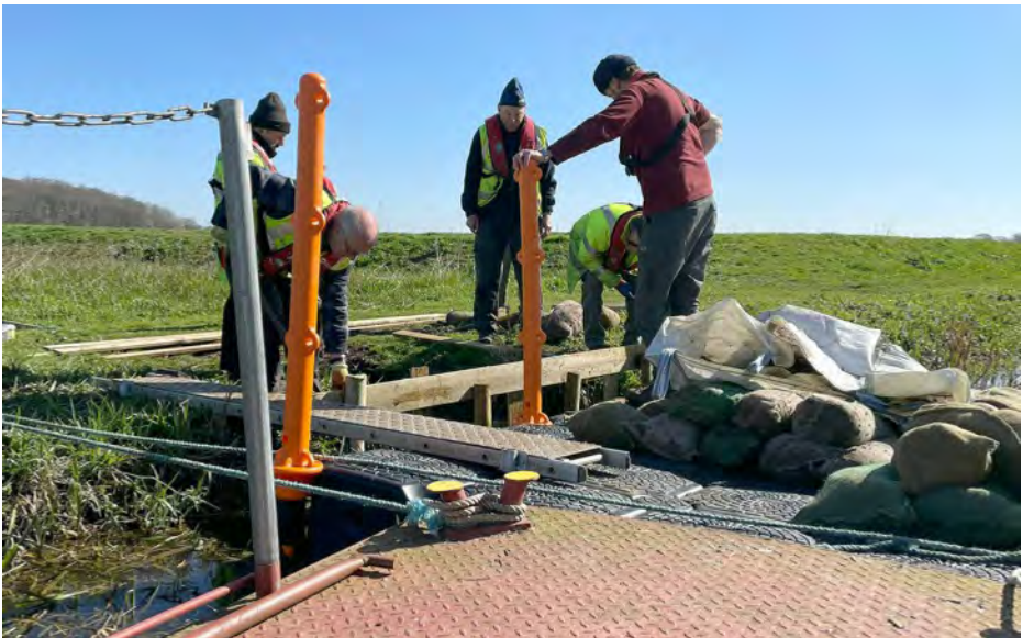
Below. Bank repairs taking place near Gardham Lock on the 4th April 2023
