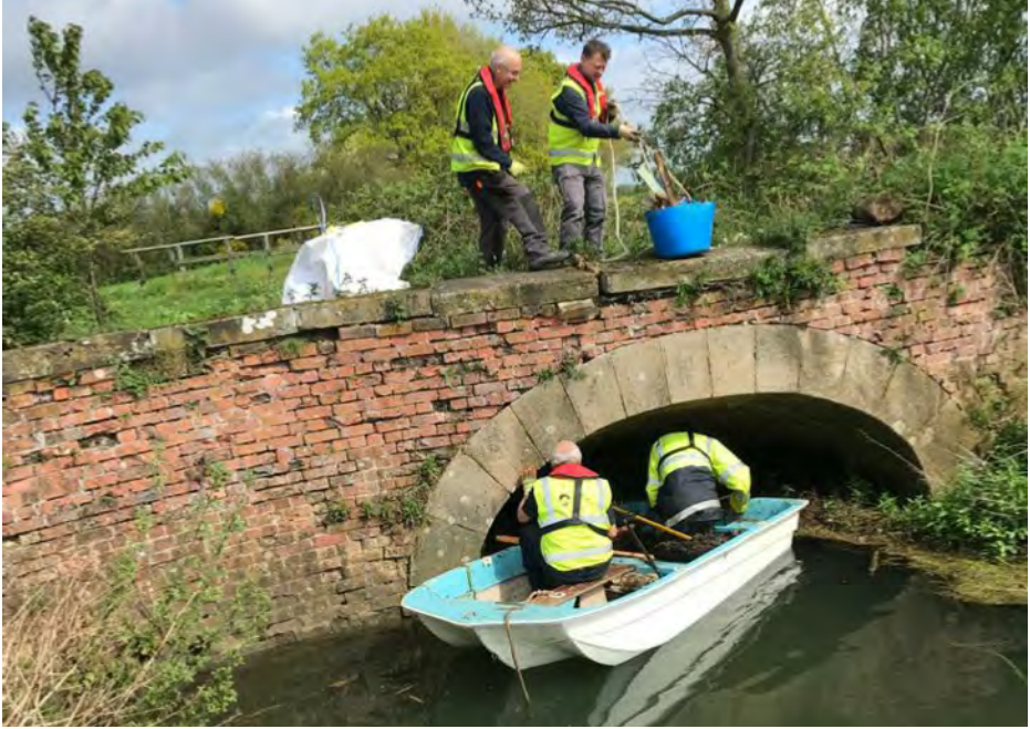
Above: Clearing debris out from the syphon above Thornton Lock on the 9th May 2023
